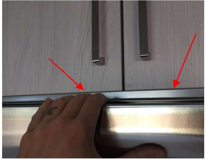
Photo 76-360(2): Kitchen- cabinet doors above fridge drag during operation
