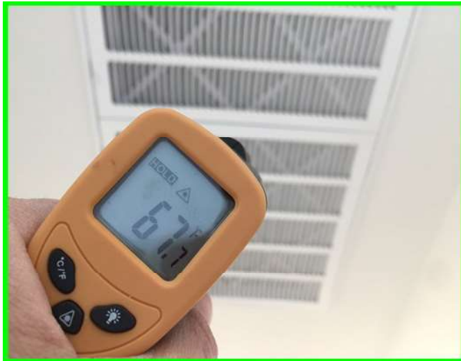
Positive Photo 21-005(1): Inlet temp
