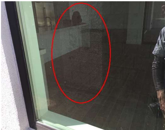
Photo 17-120(5): Paint overspray on multiple windows
