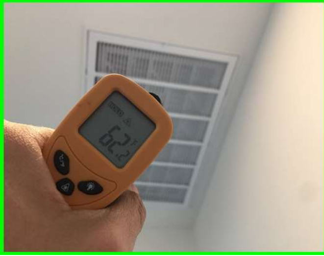
Positive Photo 21-005(3): Inlet temp
