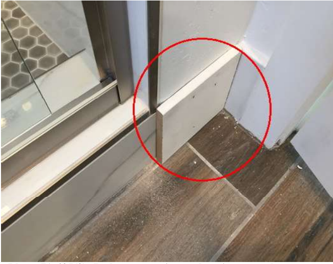
Photo 71-435(9): Bedroom ensuite- end grain exposed; no return
