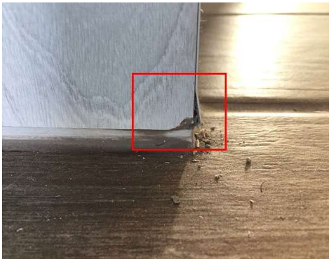
Photo 76-360(11): Kitchen- damage at fridge enclosure
