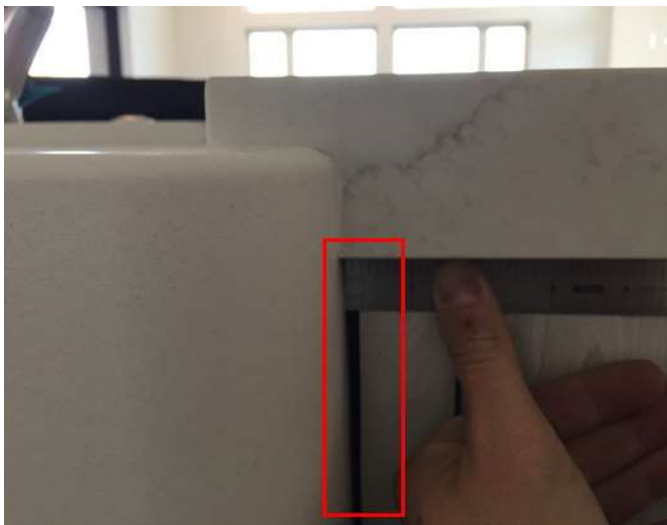
Photo 76-360(5): Kitchen- gap at sink basin
