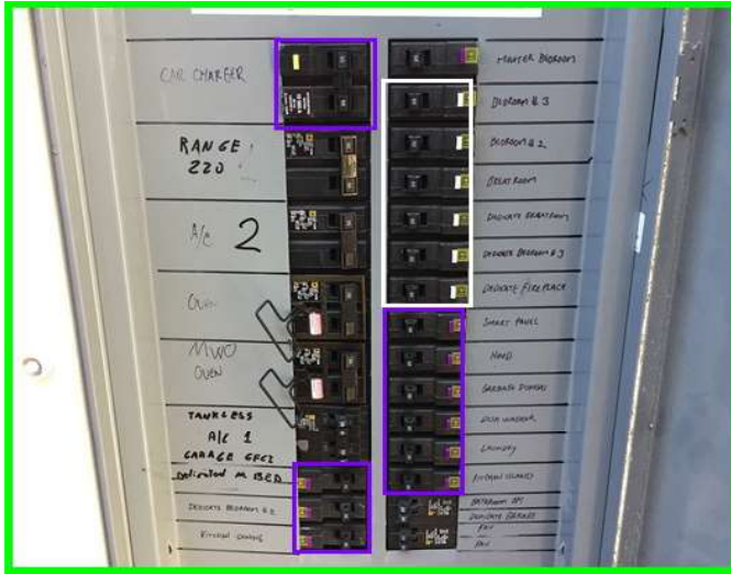
Positive Photo 55-009(1): Purple = GFCI/AFCI combo; White = AFCI
